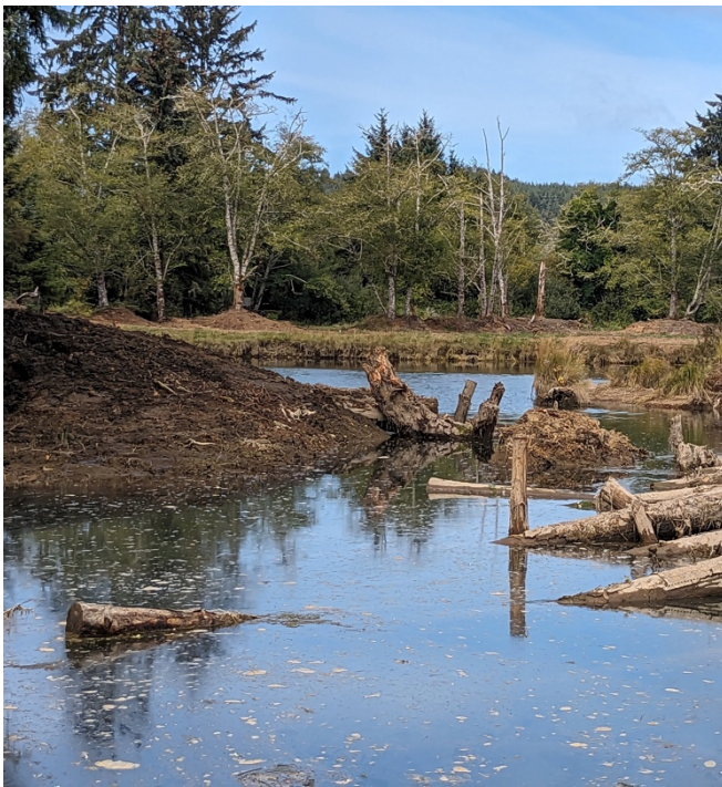
Mound graded to provide elevated topography in a restoration project. Siletz Bay, Oregon, USA. Photo by Fran Recht.
